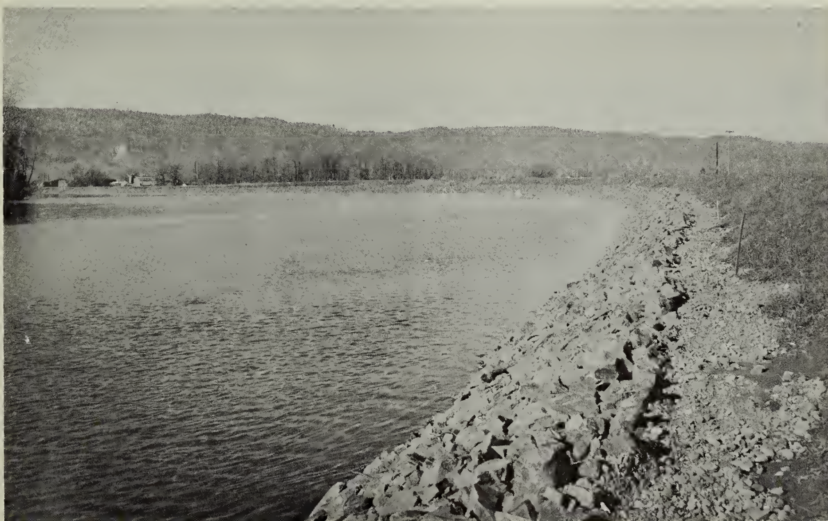
Photo 29.--This portion of the Clatskanie River bank has been protected by rock riprap, Oregon, 1962. SCS photo
